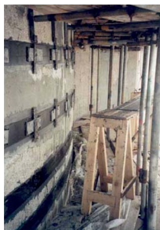
Figure 3. The proposed method of securing the laminates to the tower whilst the adhesive cured
