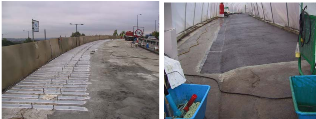
Figure 2. CFRP Laminates Bonding/Strengthen Deck Edge Cantilever (left) CFRP Wet Lay-up/Strengthen Deck Edge Cantilever (In Polythene Tunnel) (right)
